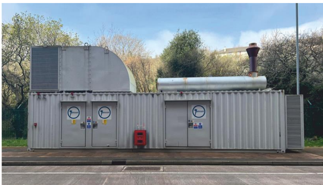
Graphic 3.12: A typical emergency diesel generator
