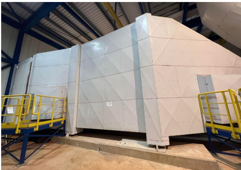
Graphic 3.8: A typical (insulated) induced draft fan within cabin
