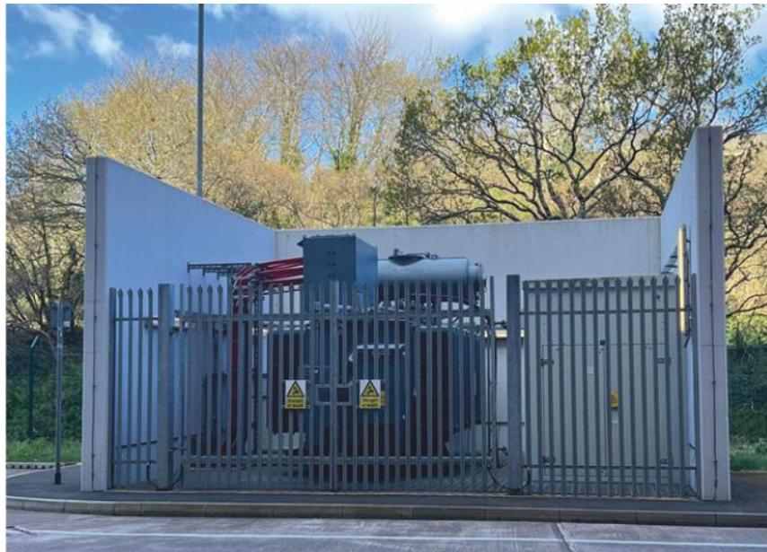
Graphic 3.11: A typical mains transformer compound
