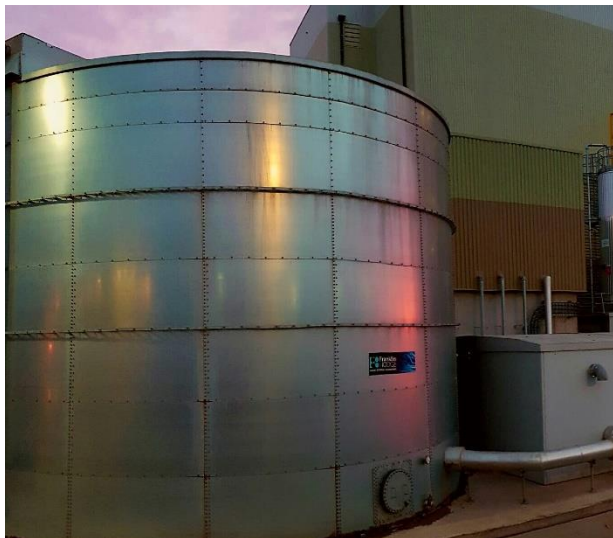
Graphic 3.2: A typical fire water tank
